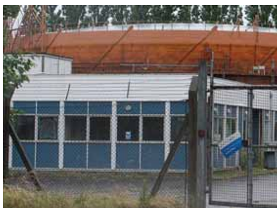
Poorly maintained boundaries in older developments (example from Sunninghill).
